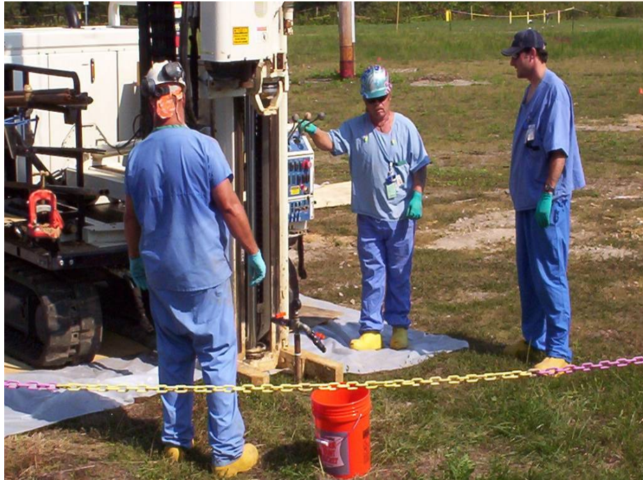
Oxidant is injected into the X-701B Groundwater Plume Area on East Side of Plant to Chemically Break Down Contaminants (Primarily trichloroethylene, or TCE)
